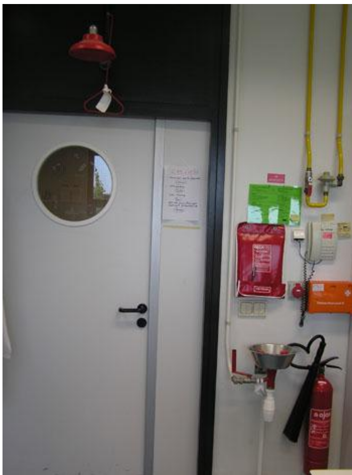
Emergency shower, eye shower, fire blanket, first-aid kit and fire-extinguisher in a laboratory.
